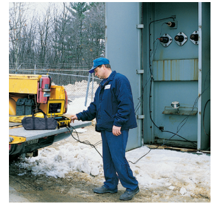
Measurement on a 2,000 kVA three-phase transformer in the field
