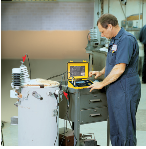
Measurement on a transformer in the workshop
